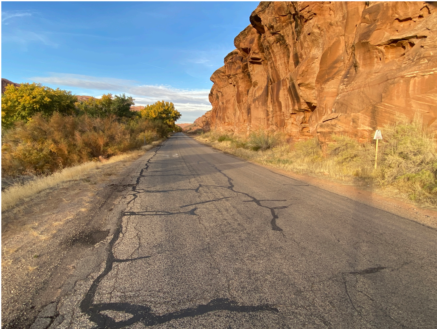
Kane Creek Road looking upstream. SWDs are along the bedrock cliff & ledges. There is a buried gas pipeline in this easement corridor. The destination of this fuel is the downstream solution mining facility operated by Intrepid Potash. The Colorado River reached these bedrock cliffs during the 20th century pluvial, in 1884 and in 1862.
