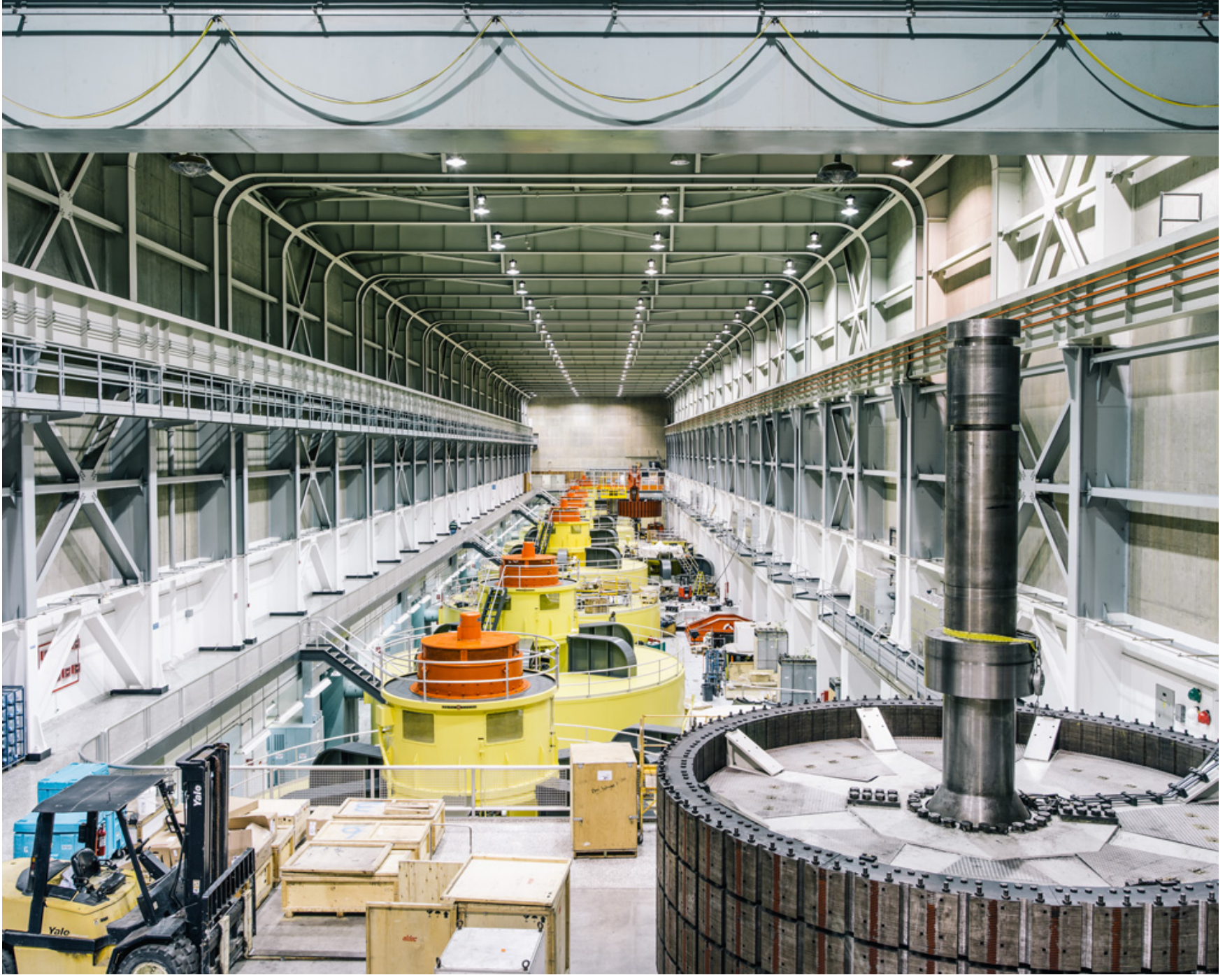
Turbines inside the Glen Canyon Dam, a great source of electrical power for the American Southwest.
